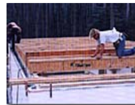
The outstanding compressive strength of TF walls allow for the installation of floor systems before pouring.
